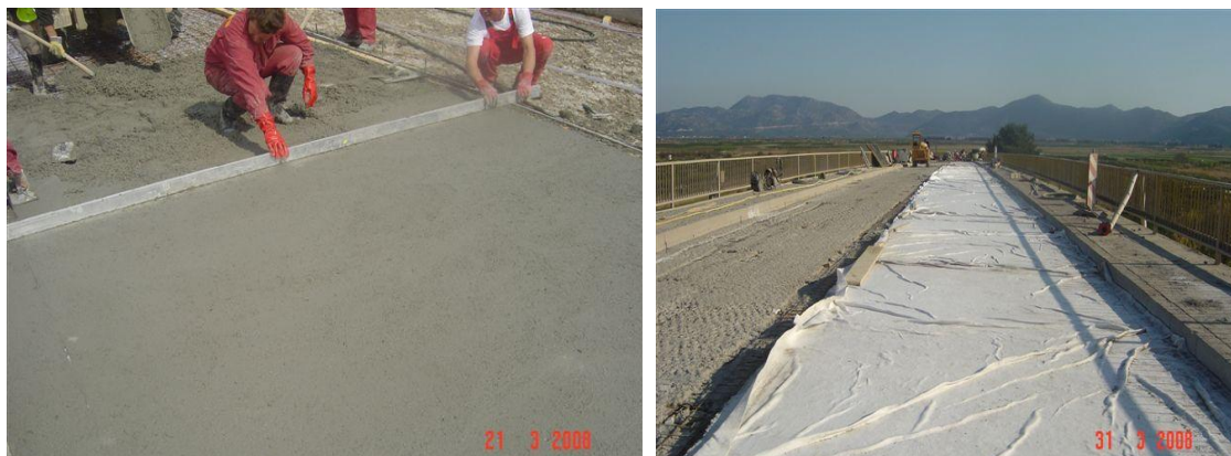
Fig. 6. Surface finishing of bridge deck (left) and curing of the concrete placed (right)
