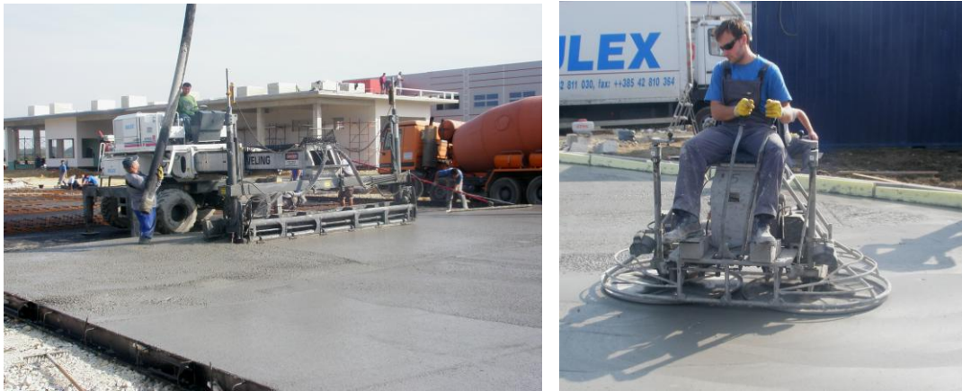
Fig. 3. Concrete placement in the pavement by concrete finisher (left) and surface finishing (right)
