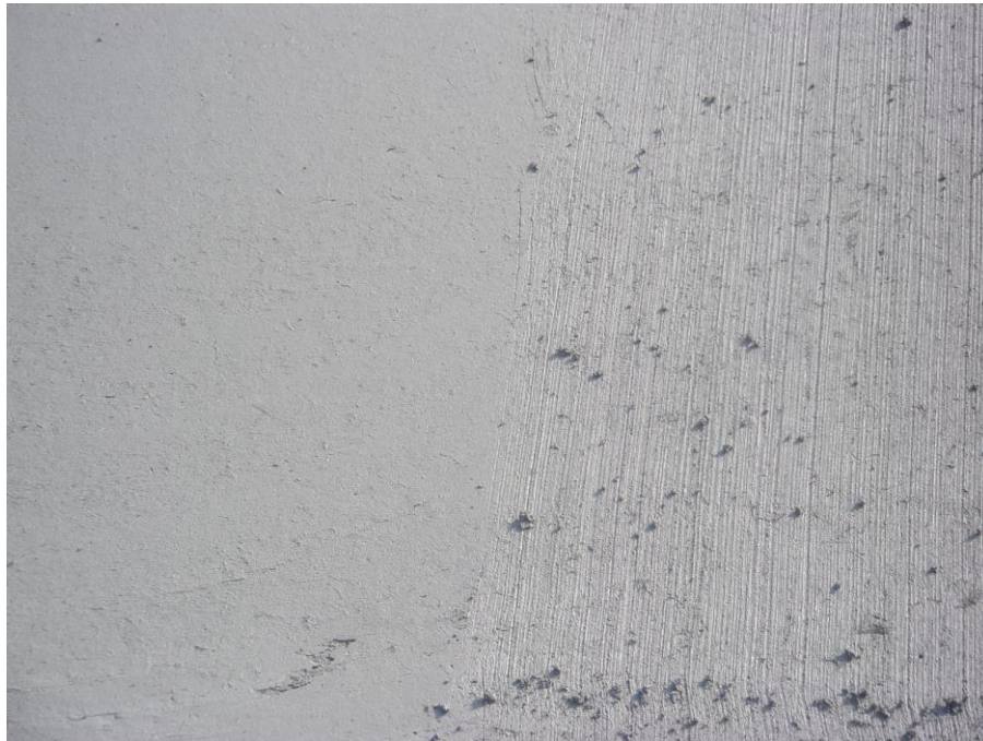
Fig. 4. Final appearance of the concrete pavement without being swept (left) and after being swept (right)
