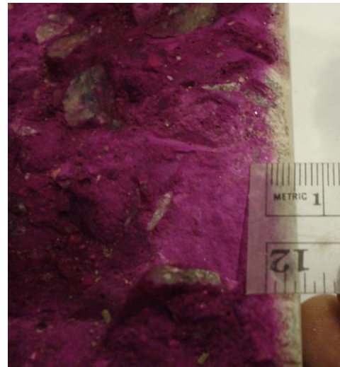
Fig. 7. Another View Showing Carbonation Depth in a Concrete
