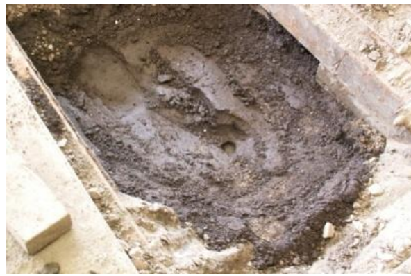
Fig. 7. Very clayey soil, not suitable for compaction
