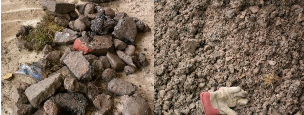
Fig. 2. Trench arisings separated by size: on the left the larger material that will need to be crushed, on the right the finer material
