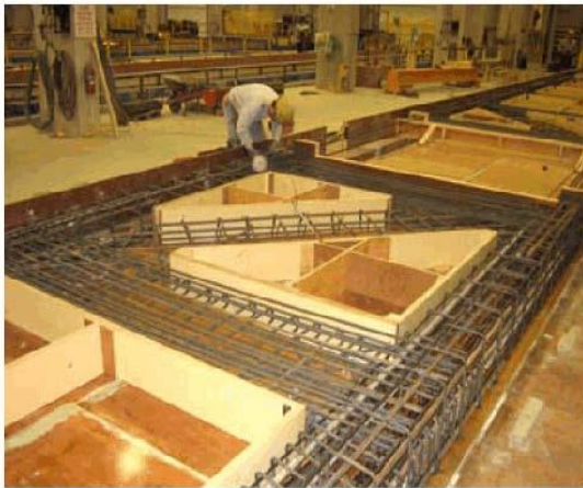
A Spancrete employee at the Valdres plant works on production of the ER Post™ Structural System.
