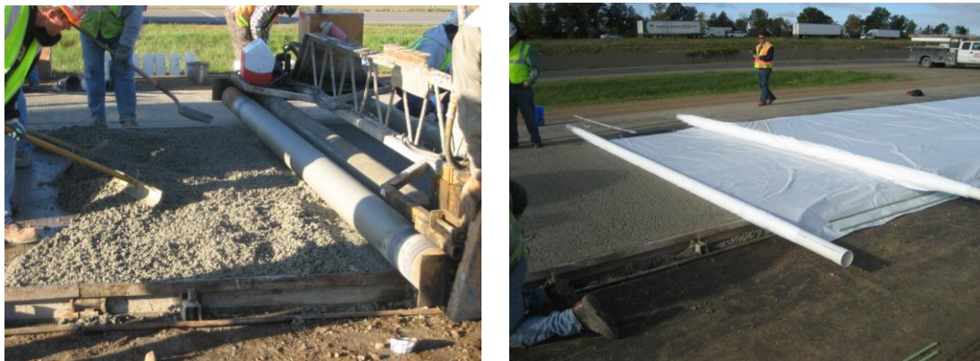
Fig. 3. (a) Placement of Pervious Concrete Overlay using Roller-screed. (b) Completed Surface of Overlay and Covering with Two Layers of Plastic
