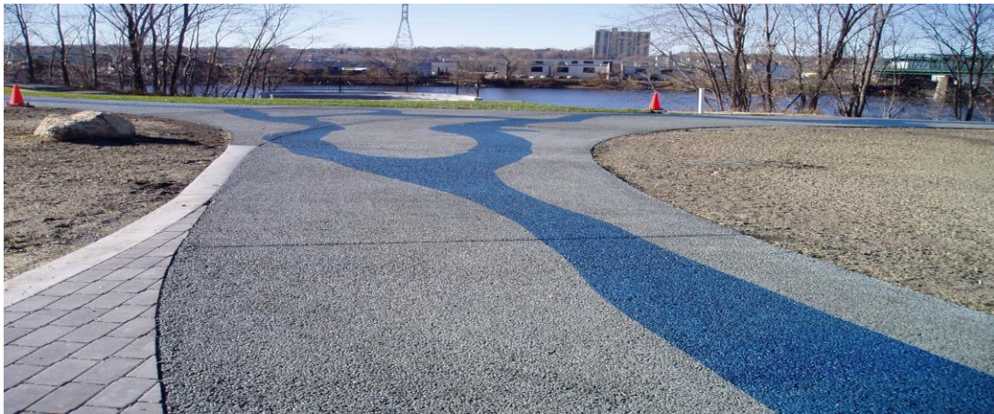
Figure 17. Pervious Concrete, integrally colored with stain applied to the surface to create an effect symbolic of two rivers converging. Minneapolis, Minnesota
