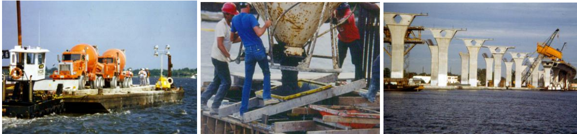
Fig.9-11 Mass concrete barged to location for a new US 1 bridge structure over an ocean inlet.
