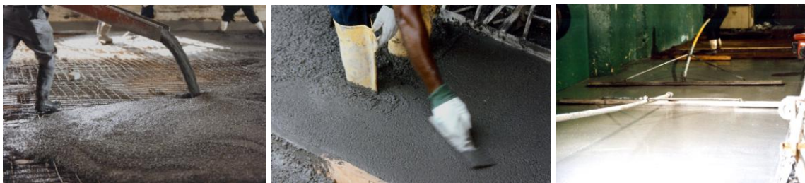
Fig.24-26 Full depth waste transfer floor replacement with 20% silica fume HPC doubled life.
