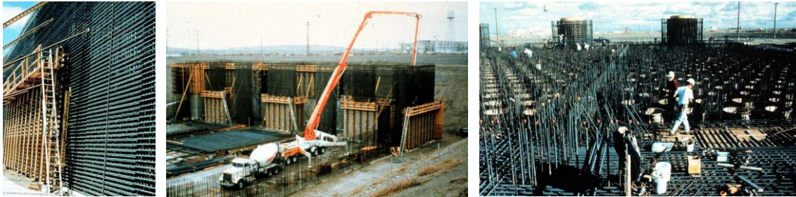
Fig.2-4 Low heat of hydration mass concrete for the Hanford Nuclear Site in waste deposit.
