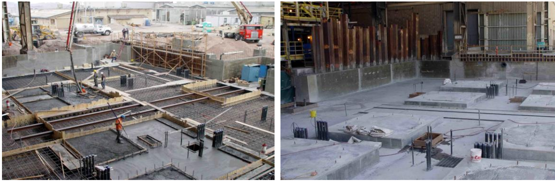
Fig.27-28 Nevada titanium plant retrofit with ultra-durable, high silica fume percentage HPC.
