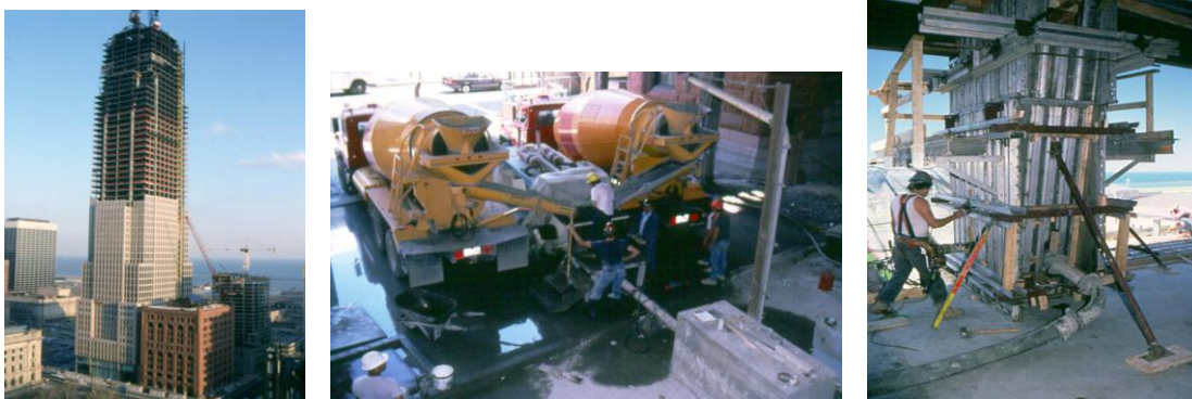
Fig.18-20 Full height single stage concrete pumping and filling columns from the bottom up.
