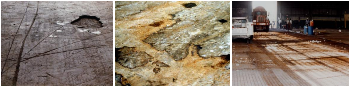
Fig.21-23 Waste transfer floor deterioration within 3 years of use are ready for replacement.
