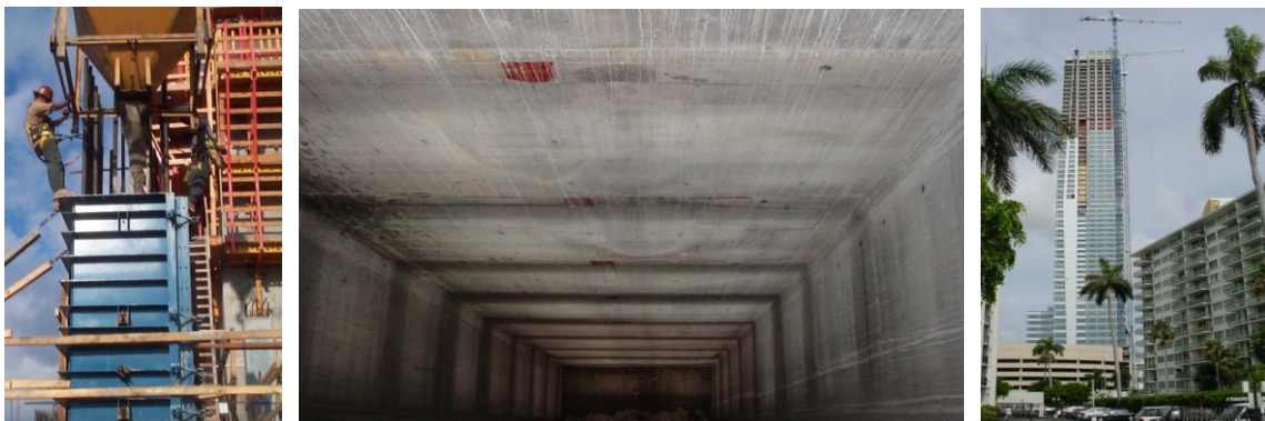
Fig.12-14 HPC column placement; internal view of elevator shaft and nearly finished structure.
