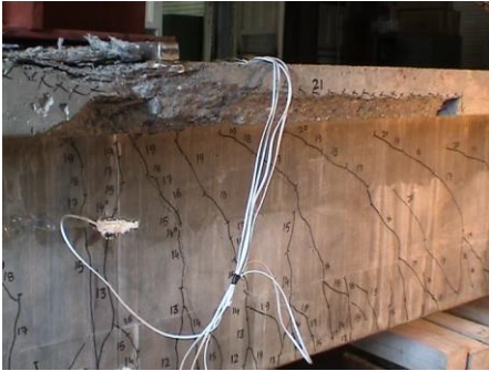
Figure 7 – Failure of PSCC1 T-beam
