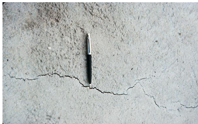
Figure 3. A typical plastic shrinkage crack (Cement Concrete & Aggregate, 2002, ( http://www.astm.org/DIGITAL_LIBRARY/JOURNALS/CEMENT/TOC/2412002.htm ))
