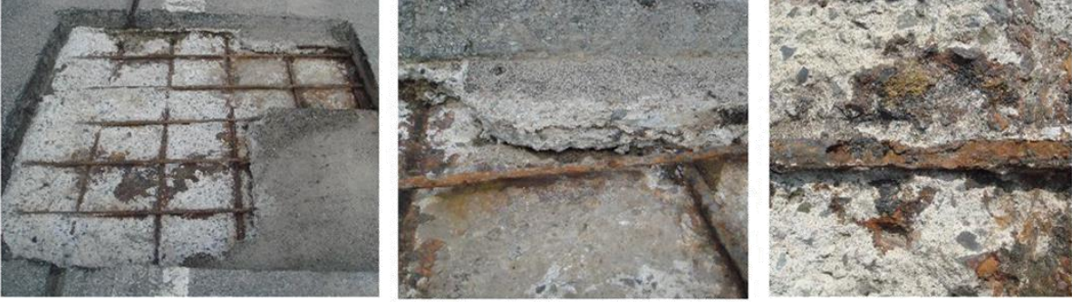
Photo 1. Corrosion of Rebar and Spalling of Concrete on the Upper Surface of Floor Slab
