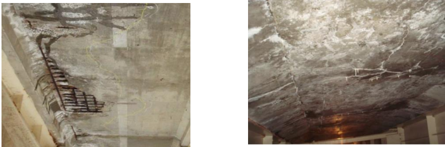
Photo 2. Corrosion of Rebar and Spalling of Concrete on the Lower Surface of Floor Slab
