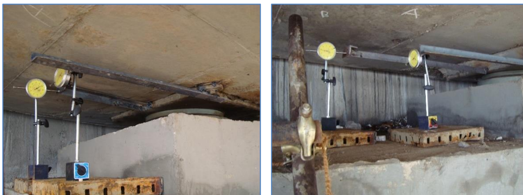
Figure 11. Placement of dial gauges for longitudinal and transverse movement of Free Type bearing
