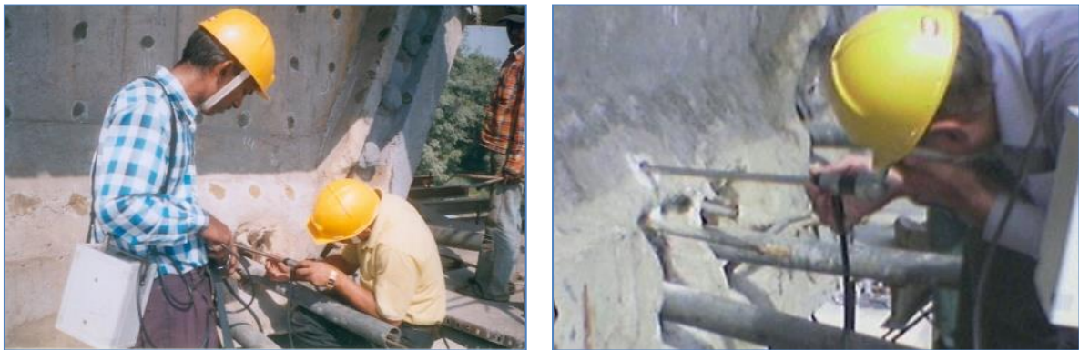
Figure 6. Examination of honeycombing through Boroscope around Anchorage zone
