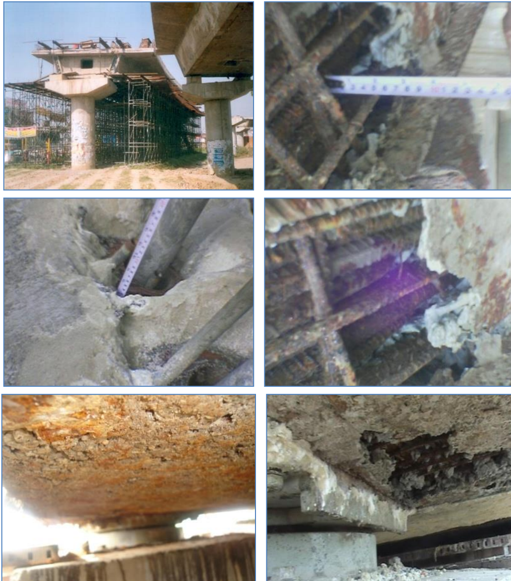
Figure 3. Views of Distressed Span P2-P3 on Outer Carriageway
