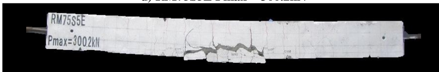
Figure 6. Final failure pattern for RM75S beams
