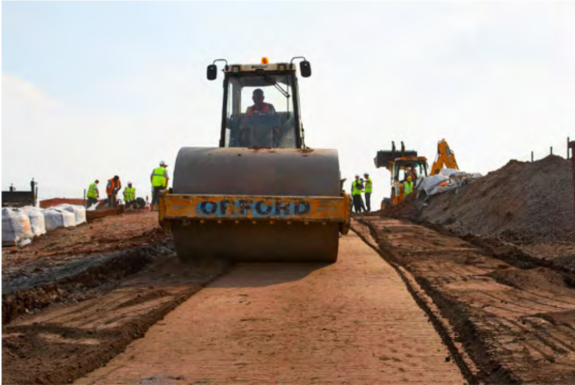
Figure 2. Compacting of the blended soil and the binder using the 10-tonne roller
