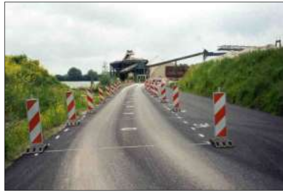
Figure 2 Overview of the prototype test site.
